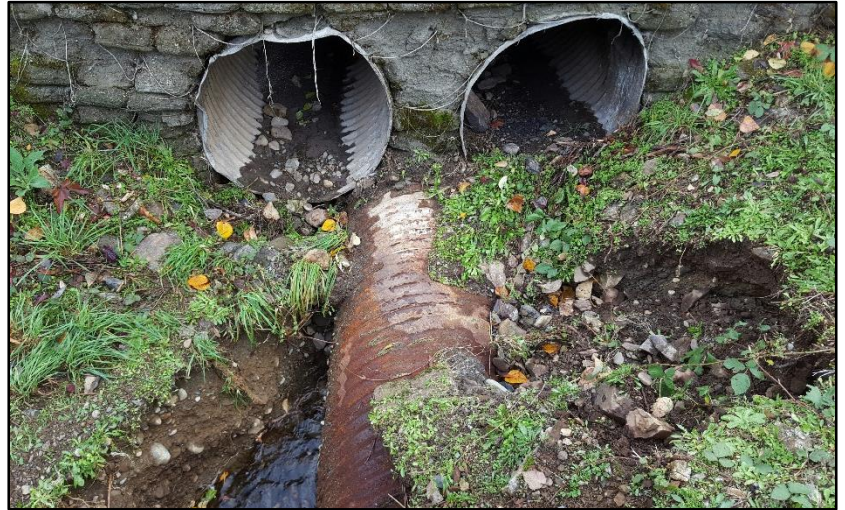
Figure 3. Lake Ida Ann Overflow Culverts and Failed Drain Culvert
