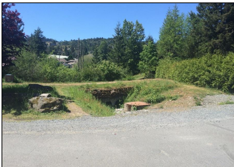
Figure 1. Open air drain ditch seen from Ashley Place
