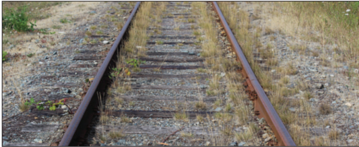
The Island Rail Corridor has been left to deteriorate since passenger service ended in 2011. (Black Press Media file photo)
