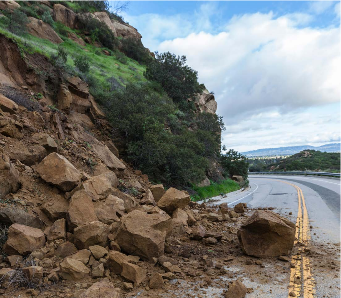
Example of landslide on highway.
